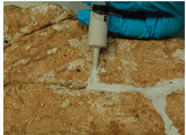
Fig. 4. Treating the back part of the wall painting by injecting inert synthetic mortar to stabilise the adhesion of the fragments.
